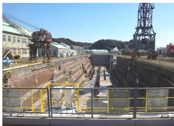
Fig.4 Present condition of the dry dock made by bricks, (Photo by author in 2014). Dock gate is at the back. Arm of the crane of right hand side is taken off and covered by rust,
