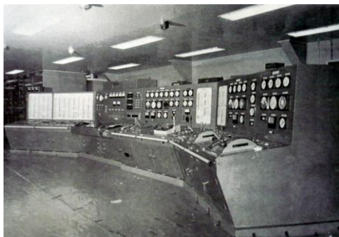
Fig.10 TOYAMA Engine Control Room (1)
