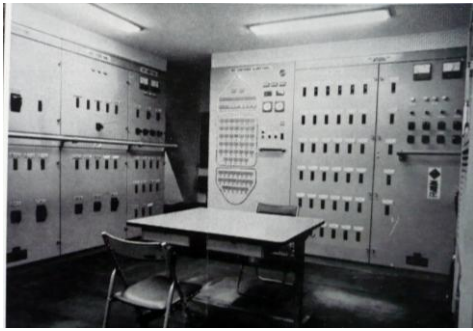
Fig.7 HAKONE MARU Engine Control Room
