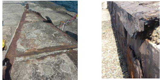
Photo 6 Corrosion / deterioration of the exposure steel materials part of destroyer (YANAGI)
