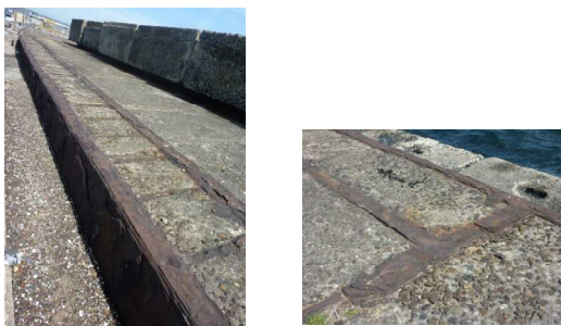
Photo 5 The side structure of destroyer (YANAGI) is photographed from the diagonal upper part (repaired)
