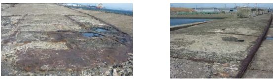
Photo 4 The top surface of destroyer (YANAGI) is photographed to the bow direction (repaired)
