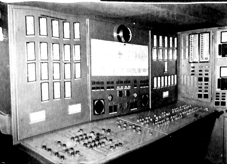
Ballast & bilge central remote control in Control Room
