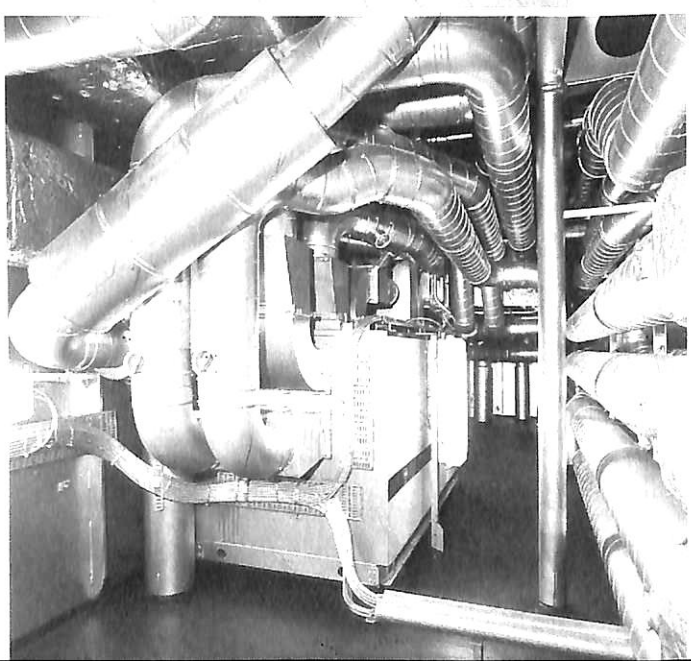
Air Conditioning Plant.
