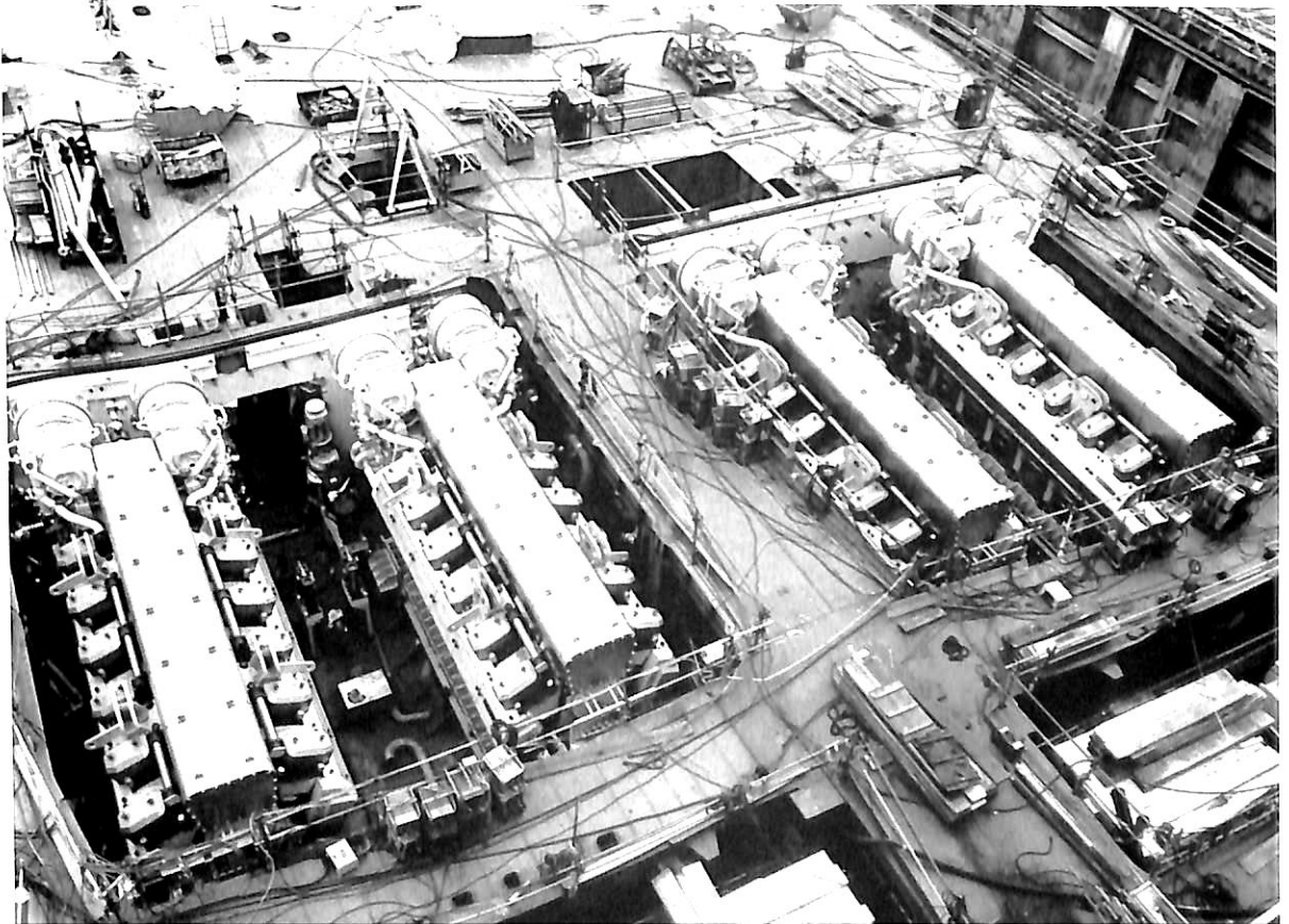
▼ "Generating sets on Tank Top"
