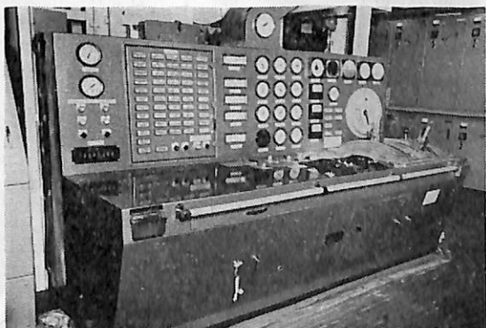
Main gauge board
